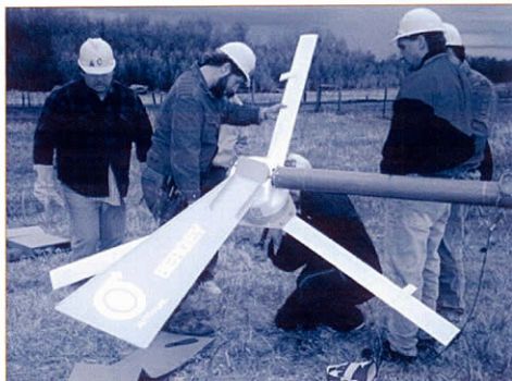
▲ Students of Assiniboine College in Manitoba install an 850 watt turbine. (Photo courtesy of Nor'wester Energy Systems Ltd.)
